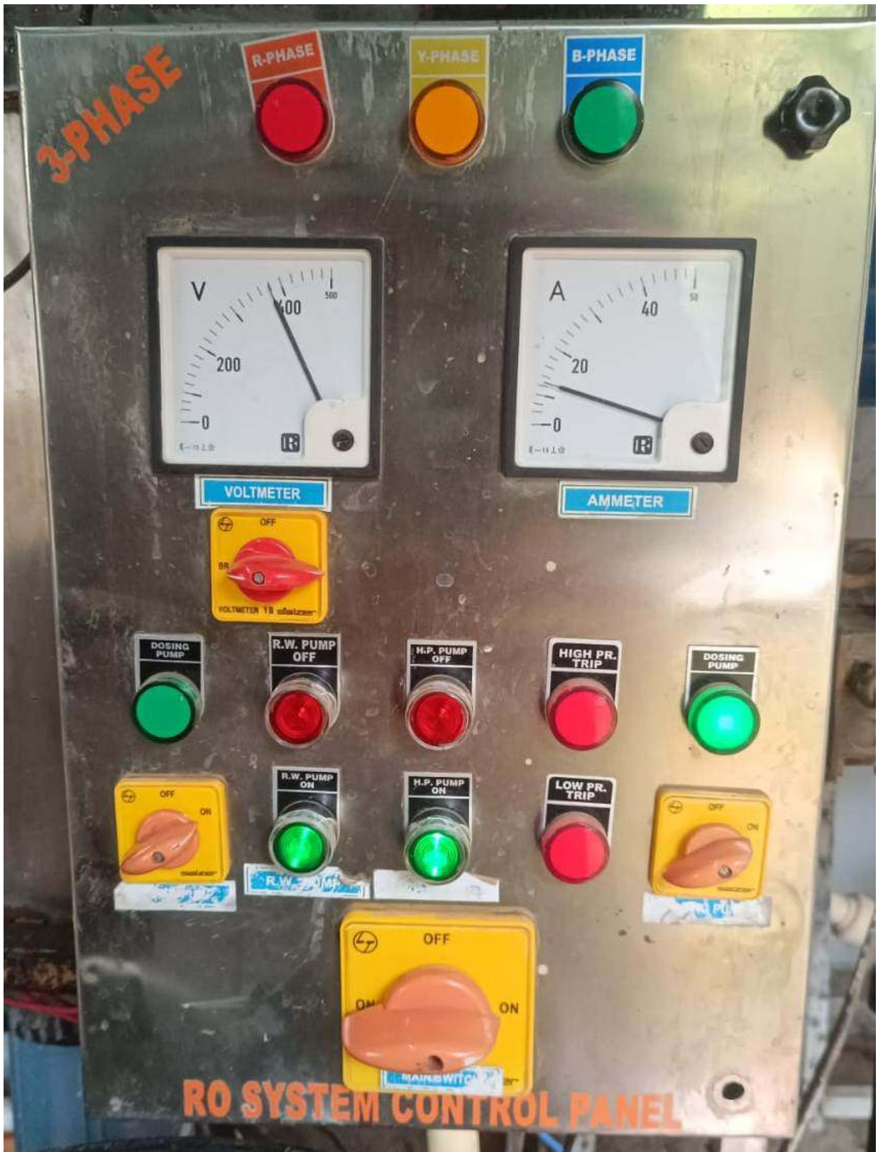
Sample photo of RO System control panel
